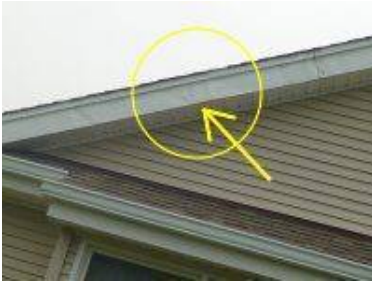
Photo X-1 One of two stressed fascia panels
