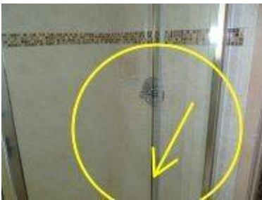
Photo X-7 Door guide missing for shower door.
