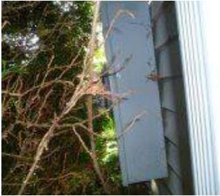
Photo X-3 Outside electric line obstructed by bushes
