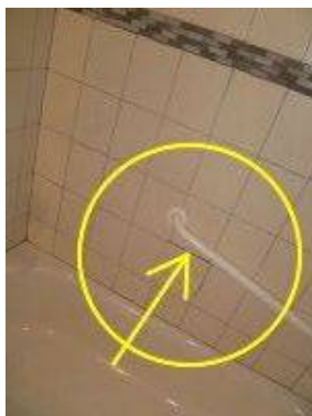
Photo X-9 Cracked wall tile in guest bathroom.
