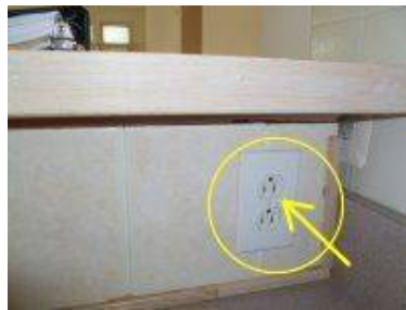
Photo X-6 Outlet mounted upside down.
