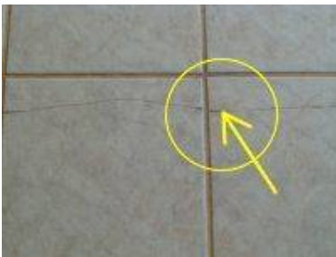
Photo X-5 Cracked floor tile in kitchen.
