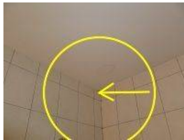
Photo X-8 Small water stain in corner of guest bathroom ceiling.
