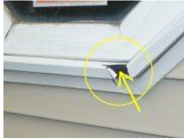
Photo X-2 Captain's window on garage side. Rotting window frame.
